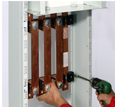
Transformer field is fastened.
