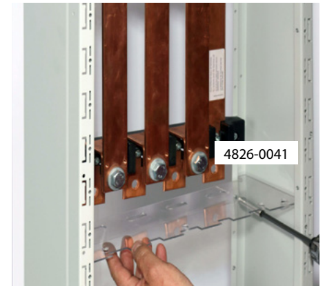
Horizontal covering is mounted below the transformer field.
