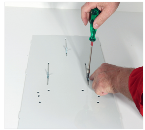
The meter plate is fastened with screws.
