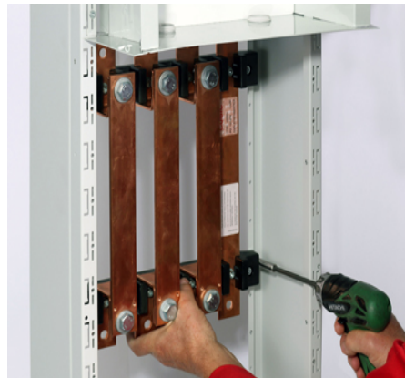
Transformer field is fastened.
