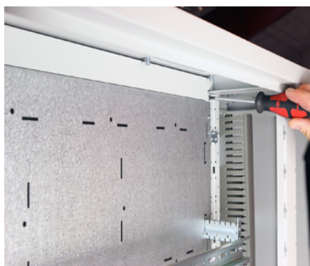
Above the mounting plates a cover is made to the busbars.
