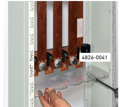
Horizontal covering is mounted below the transformer field.
