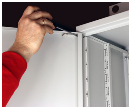
The hinge is tilted a little at the top, before the door is moved into place.
