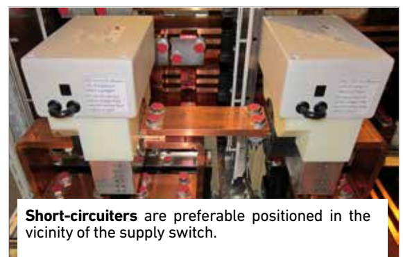
Detection devices are installed at the front of the switchgear assembly and LEDs indicate the current status of the system.
